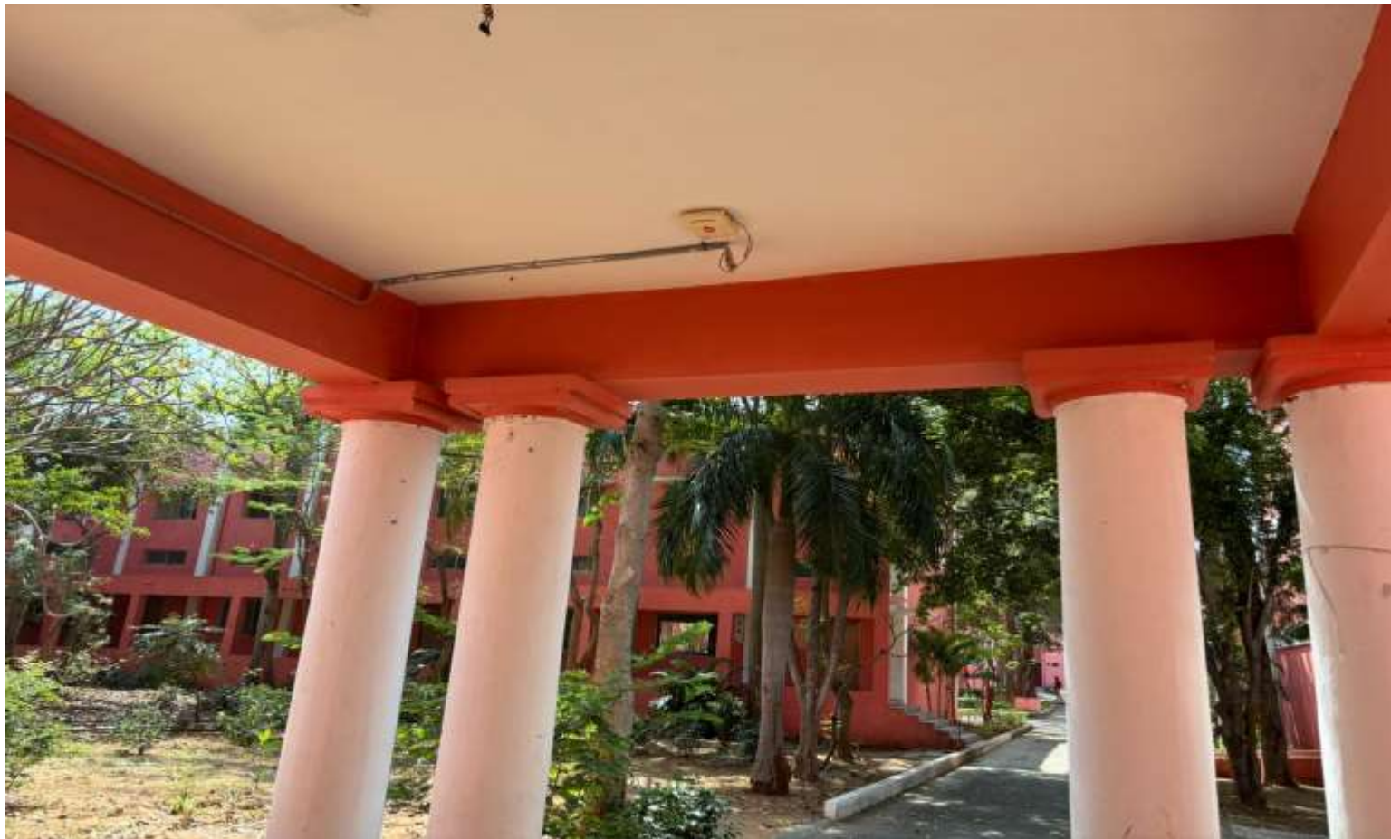
Wi-Fi Device installed at biotechnology block
